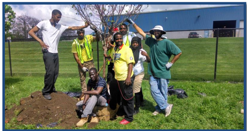
Power Corps members help install and maintain green stormwater infrastructure in Philadelphia. Power Corps supports youth workforce development and environmental stewardship and resilience. Photo Credit: Philadelphia Water Department.
